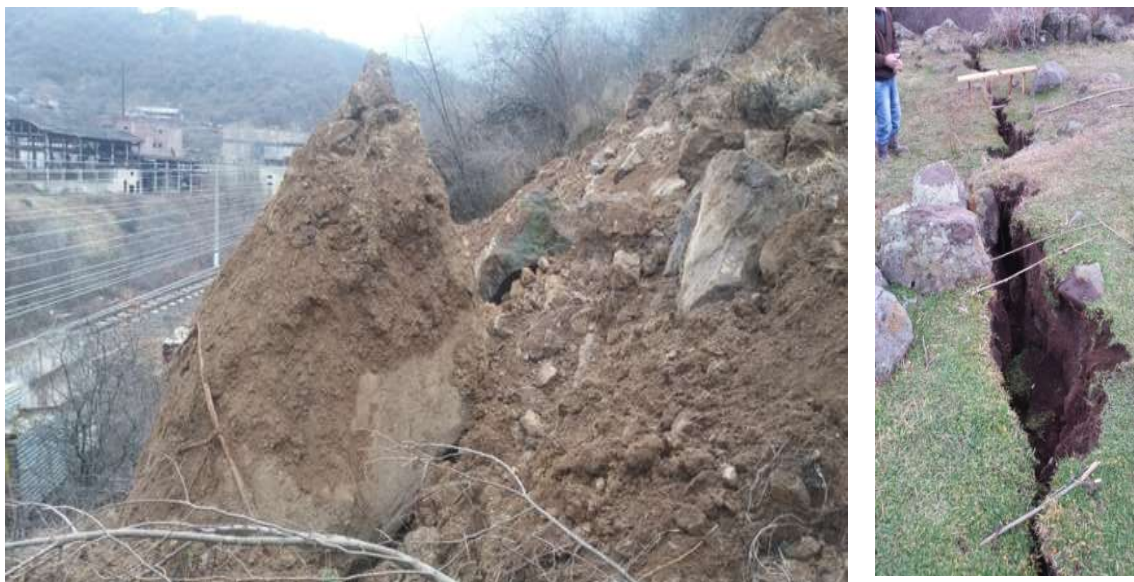
Fig. 3. The view of the Tumanyan landslide (the threat of a displaced mass on the rail) and the crack at the top, on which beacons are placed to record the movements.
